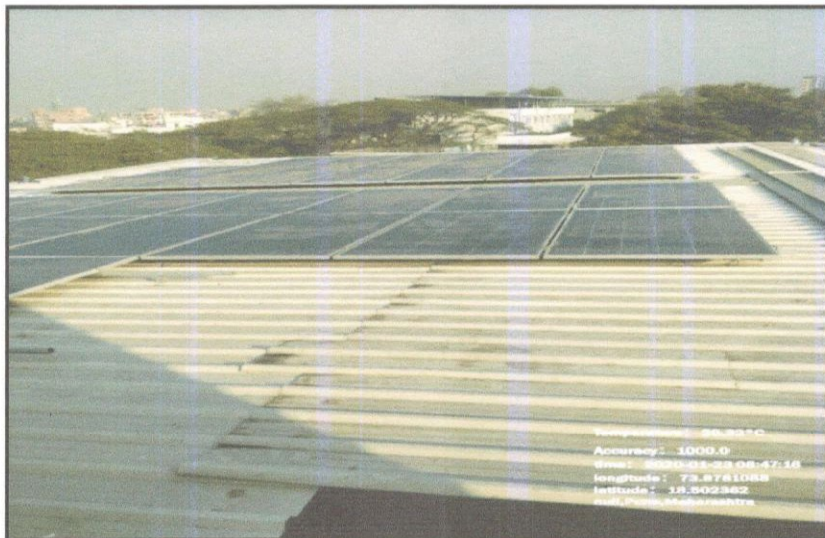
Photograph of Roof Top Solar PV Plant:
